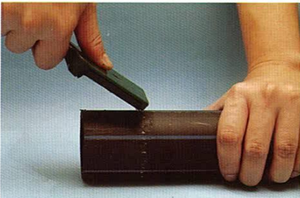
[ 4 ] Scrape the whole pipe circumference to remove all oxidation and contaminations with scrapping tool using the markings as a guide.
